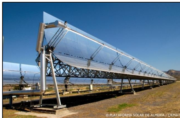
Figure 1.4. Parabolic trough collector plant at the Solar Platform of Almería.
